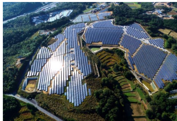
Leben Solar Hiroshima Mihara power generation facility
