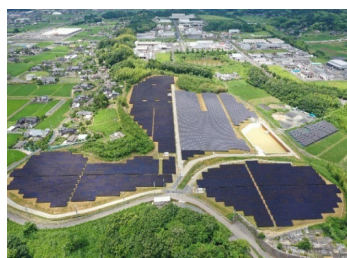
LS Okayama-Tsuyama power generation facility
