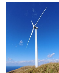
Nagasaki Tsushima wind power generation facility
