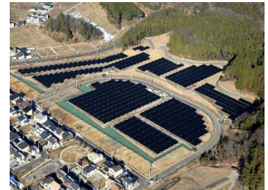
LS Hanno Misugidai power generation facility
