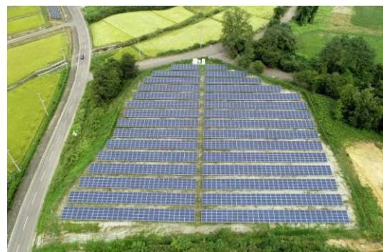
LS FUKUSHIMA KAGAMIISHI 1 power generation facility
