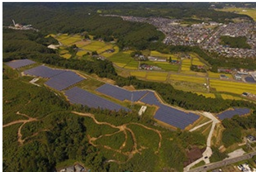
LS MIYAGISENDAI A·B power generation facility
