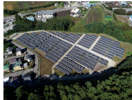
LS NAGANOSHIOJIRI power generation facility
