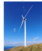
LWP Nagasaki Tsushima Power Station
