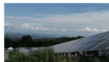
LS Tottori Daisen power generation facility (14MW)
