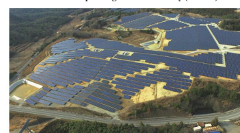
LS Mihara power generation facility (11MW)
