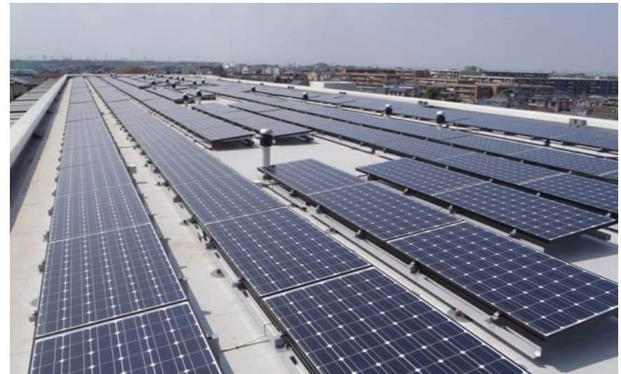
Six solar panels for each unit are installed on the rooftop of the condominium 26
