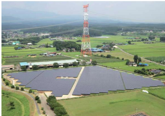
Photovoltaic power plant
